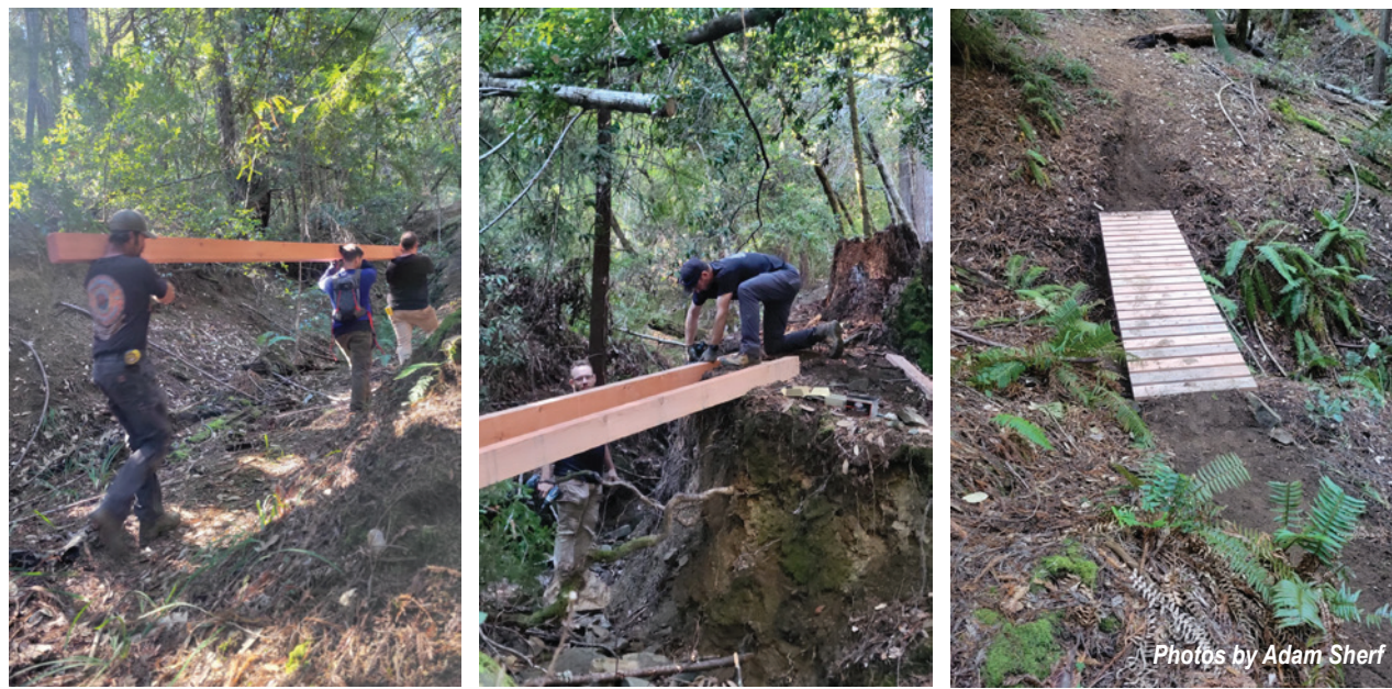
At top: A new bridge across the creek along Beaver Trail in Brooktrails, made by donated lumber from Willits Redwood Company. Above, from left: Volunteers Chris Beebe, Kyle Klesper, and Adam Winokur haul in one of many pieces of redwood lumber to make the new bridges. Volunteer Adam Sherf works on the frame for one of the new bridges, with Adam Winokur in the creekbed. This photo shows the steepness of parts of the Beaver Trail in Brooktrails.
