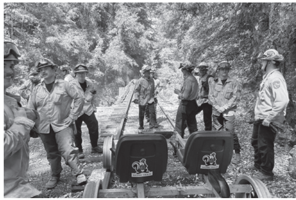
Above: Firefighters gather at the Skunk Train's Bridge 15.03, after a fire was reported July 27. Below: A firefighter wets down the burning ties on the bridge.
